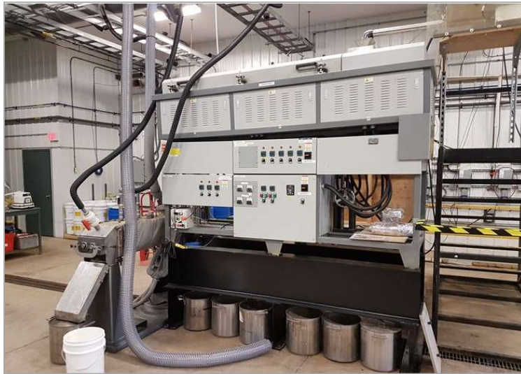
Figure 12: Screw Feeder and Pug Mill Utilized for Acid/Ore Heat and Mixing
