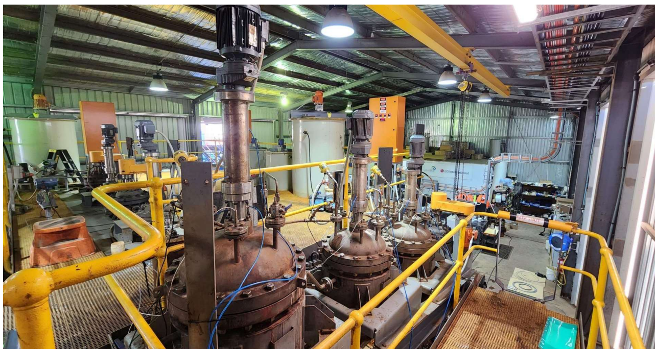
Figure 11: Demonstration Plant autoclave train
