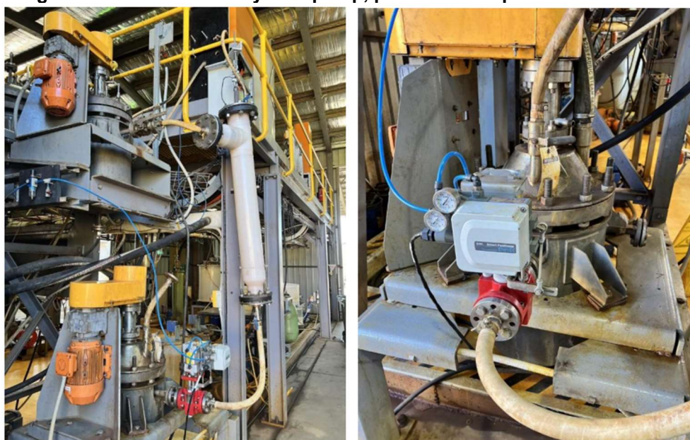
Figure 13: Demonstration autoclave discharge system – actuated pinch valve based on weight of slurry in discharge chamber
