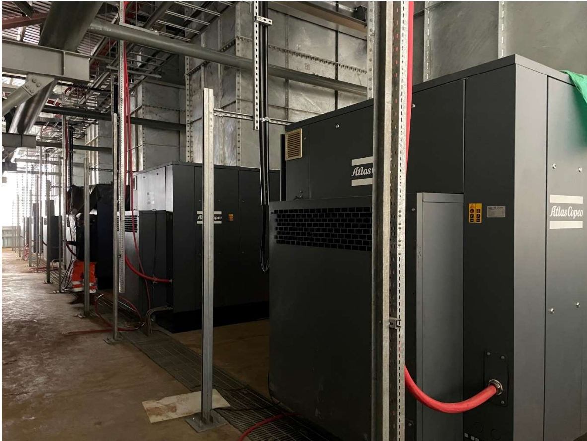
Figure 10: Air compressor room in a tailings dewatering plant with multiple 500 kW compressors
