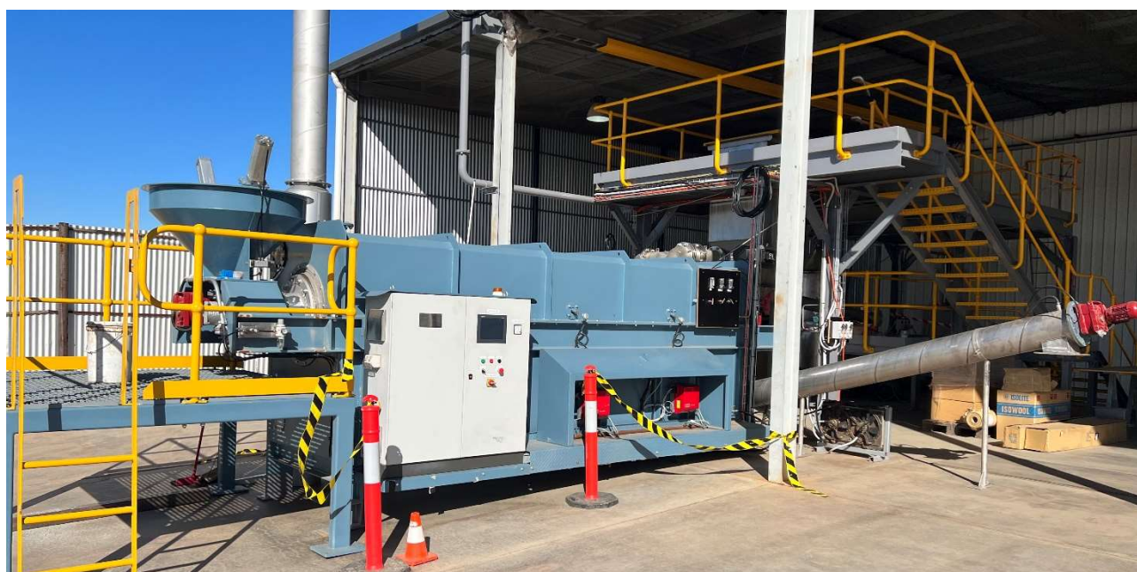
Figure 7: Demonstration Plant kiln
