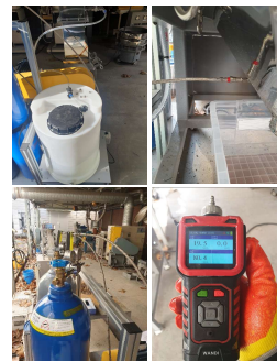
[Gas, Salt water injection system]
