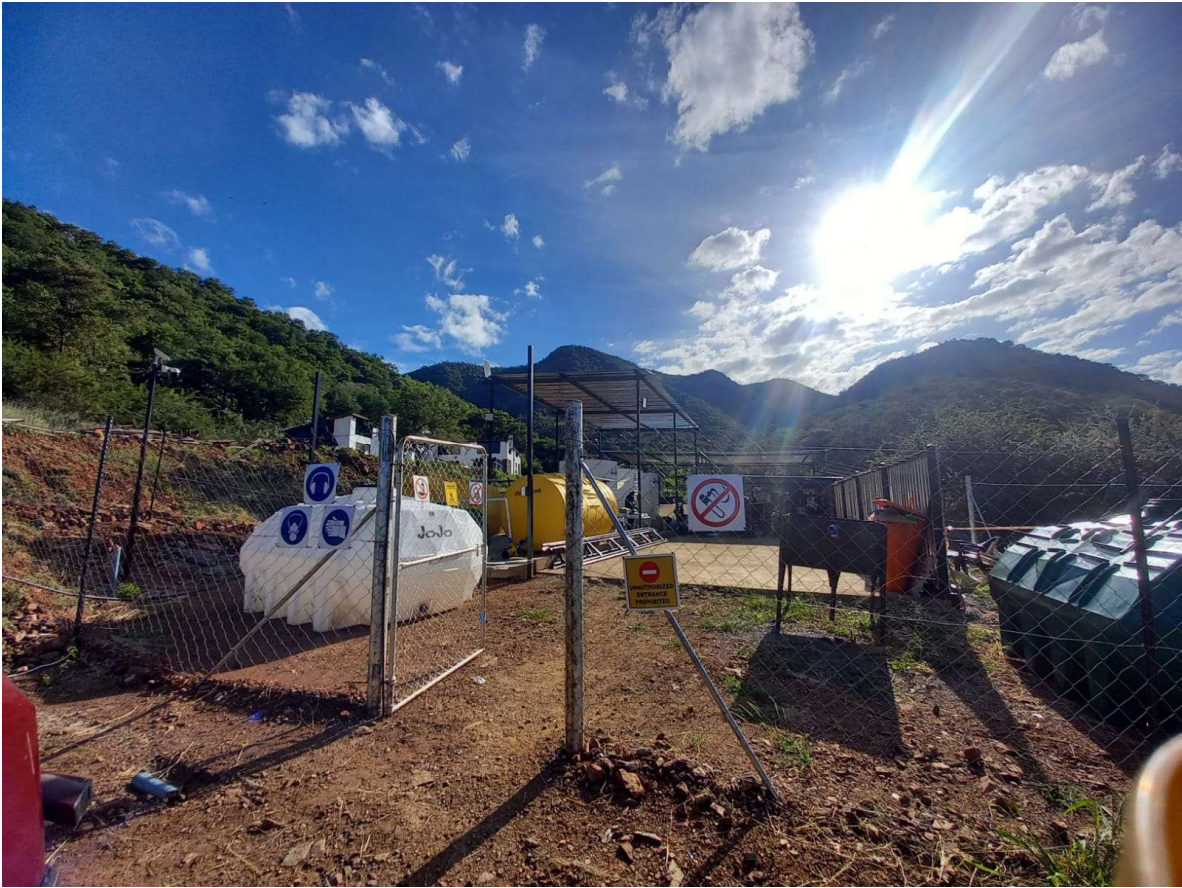
Figure 16: "Tank farm" built by the demonstration partner.
