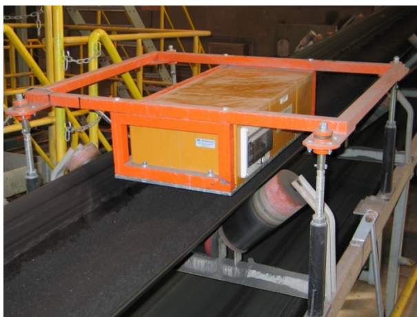
Fig.1. On-line XRF analyzer CON-X02 on the industrial conveyor PHOSPHATE ROCK AND FERTILIZERS
