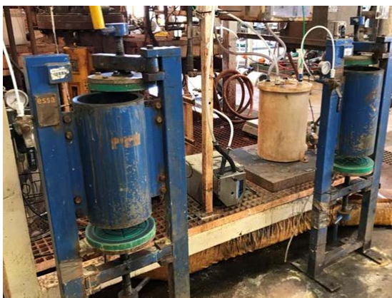
Figure 24: Pilot Plant Pot Filters
