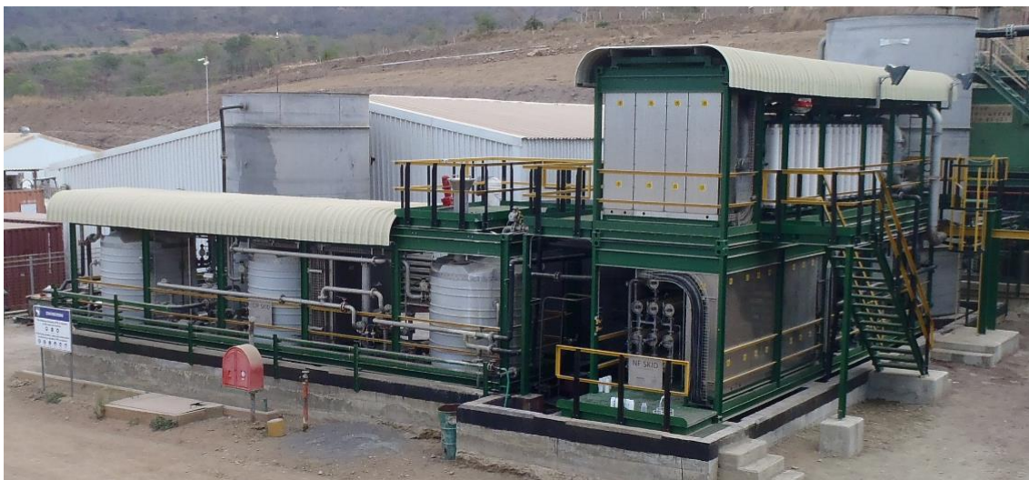
Full operational performance within 5 days from first plant feed
